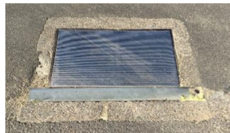
Figure 6 - Stormwater drain equipped with sediment mesh
