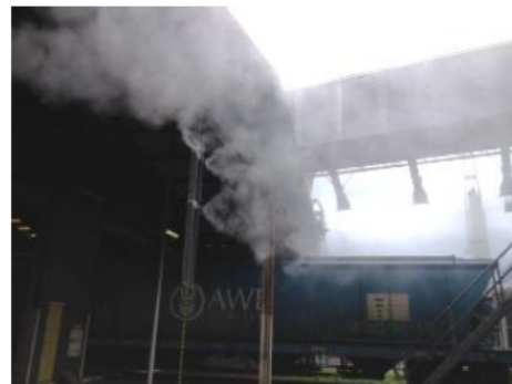
Figure 5 - Rail receival shed water spray
