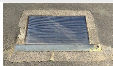
Figure 9. Stormwater drain equipped with sediment mesh
