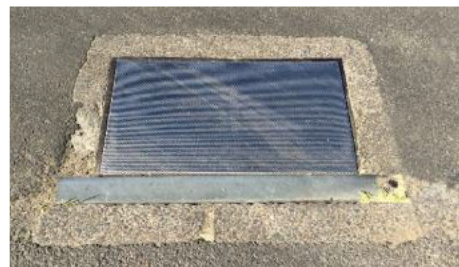
Figure 6 - Stormwater drain equipped with sediment mesh
